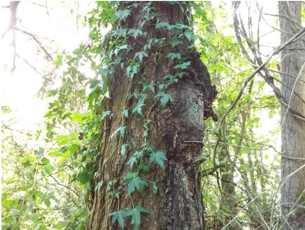
Figure 8. Large canker low on the column of the #18 tree.
